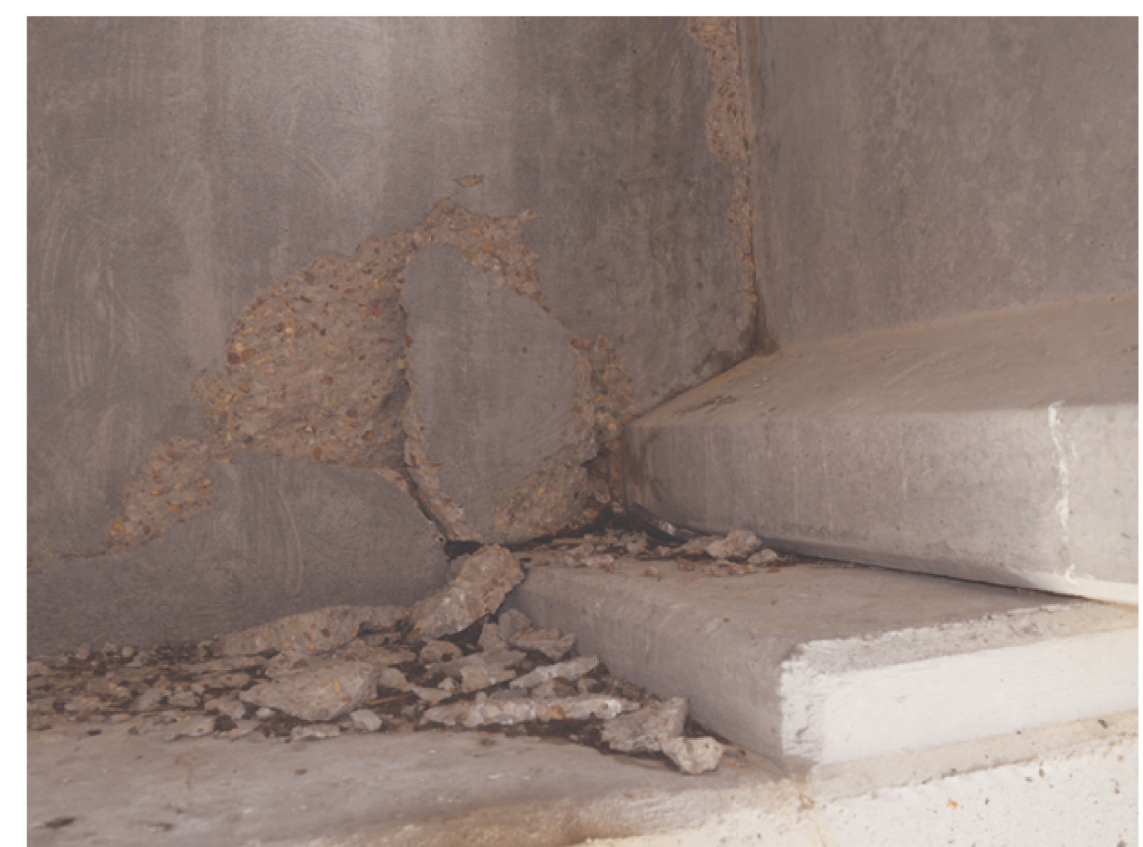
DIAPHRAGM CRACKING - AT PIER 1, SPAN 1
